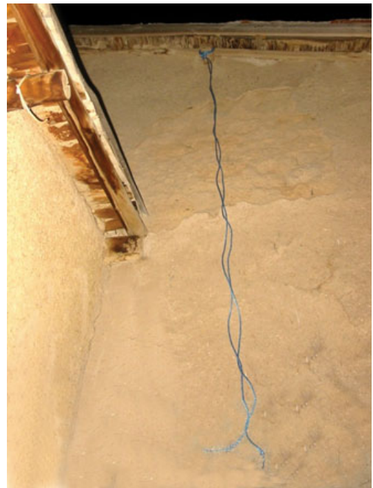
FIG. 7—Clothesline tied to a wooden beam situated over the roof at a height of 10 m (Table 2, case 4).
